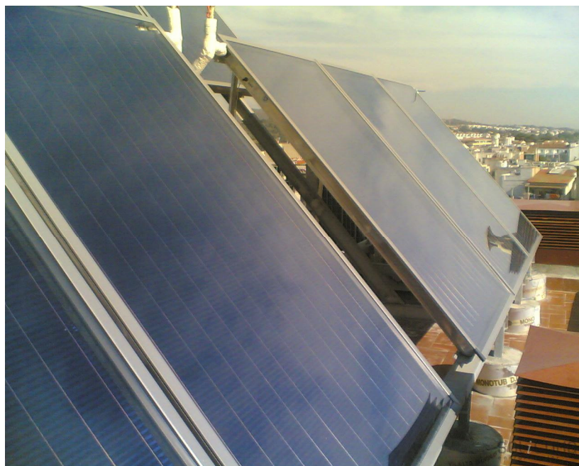
Figura 35 – Colectores solares planos [www.sunandclimate.com]
